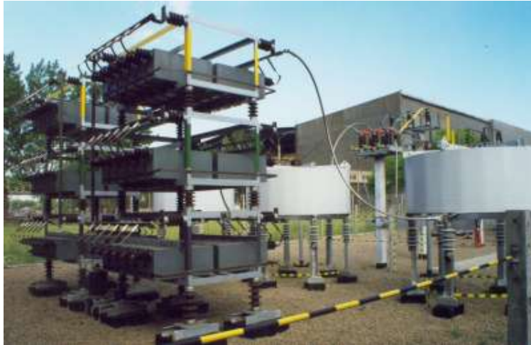
Picture of a Capacitor Bank.
